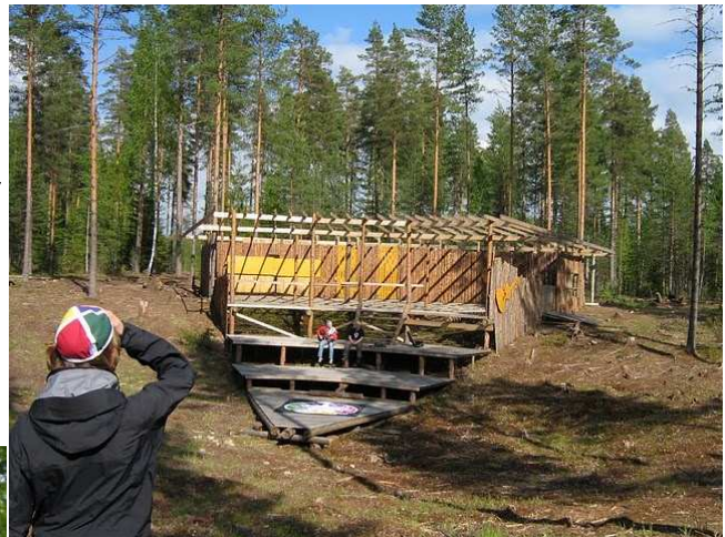
One of the many structures on the campsite – this will be a subcamp cafe.
